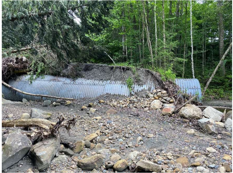
Figure 2. Large culvert exposed from road washing out in July 2024 flooding.
